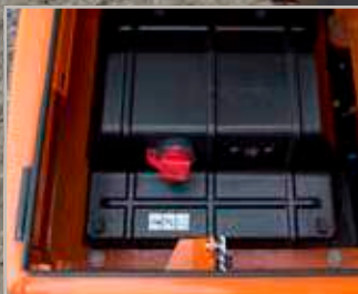
Battery cut-off switch
