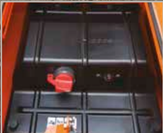
Battery cut-off switch
