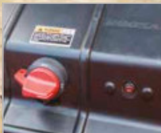
Battery cut-off switch
