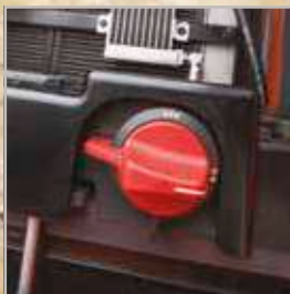
Battery cut-off switch
